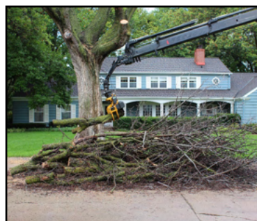
Stacking all the tree branches in one pile using the Grapple saw and crane.
